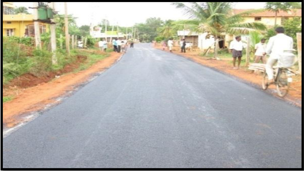
Photo 10: Rural Road: NH-206 to Basaveshwara Temple, Mattigatta Village Constructed with RBI Grade-81, Gubbi, Tumkur, Karnataka
