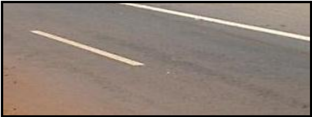
Photo 5: Close up view of National Highway Test Stretch Constructed with RBI Grade-81: Bus Bays at km 46 & 49, NH-206, Tumkur, Karnataka
