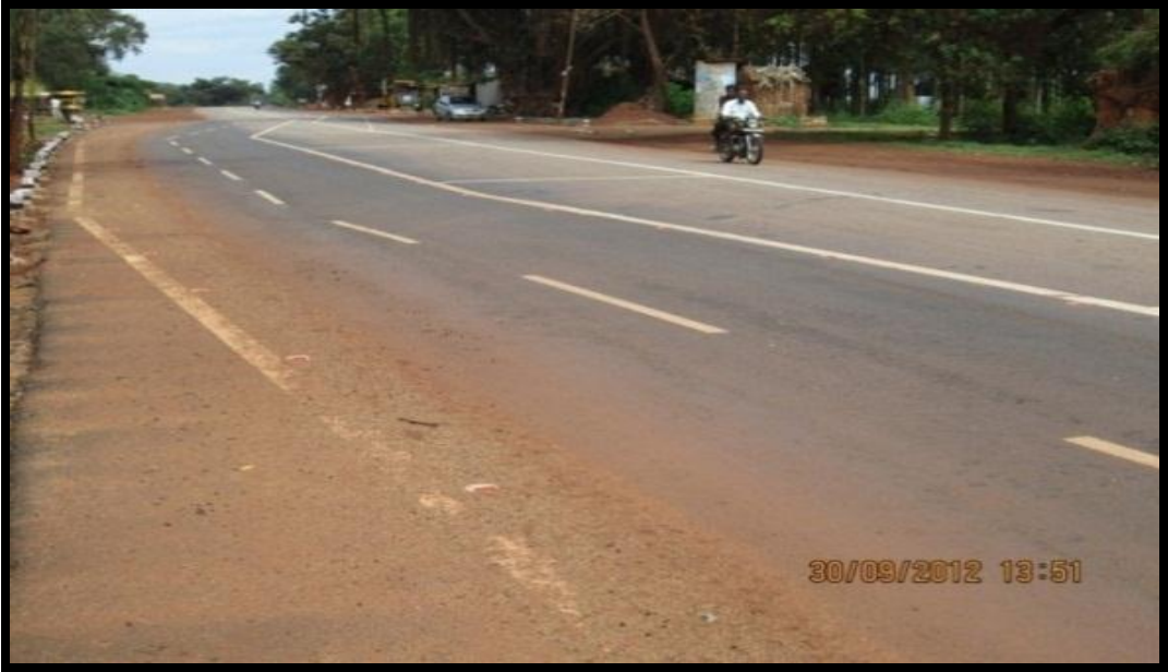
Photo 4: National Highway Test Stretch Constructed with RBI Grade-81: Bus Bays at km 46 and 49, NH-206, Tumkur, Karnataka
