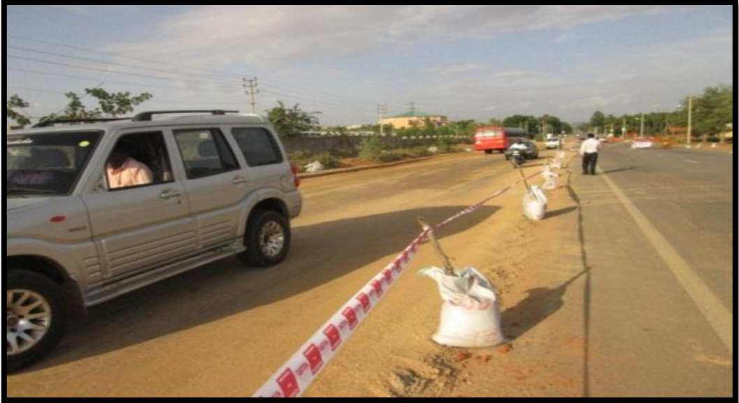
Photo 6: Temporary Diversion for Strengthening: Constructed with RBI Grade-81 km 9.30 to 9.80, NH-206, Tumkur, Karnataka
