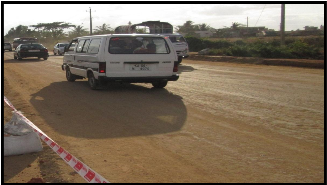
Photo 7: Temporary Diversion for Strengthening Constructed with RBI Grade-81 km 9.30 to 9.80, NH-206, Tumkur, Karnataka
