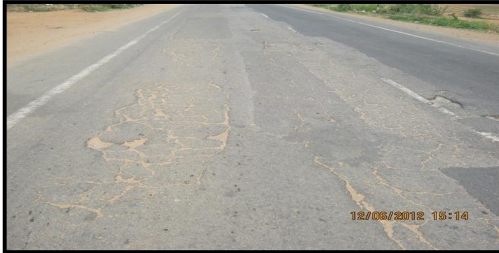
Photo 3.25: Initial view of distressed pavement
