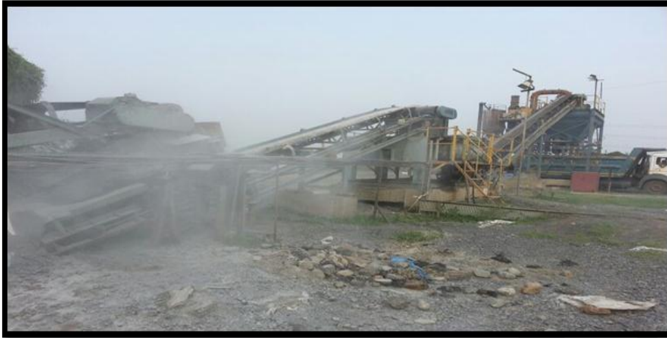
Photo 3.35: View of WMM Plant
