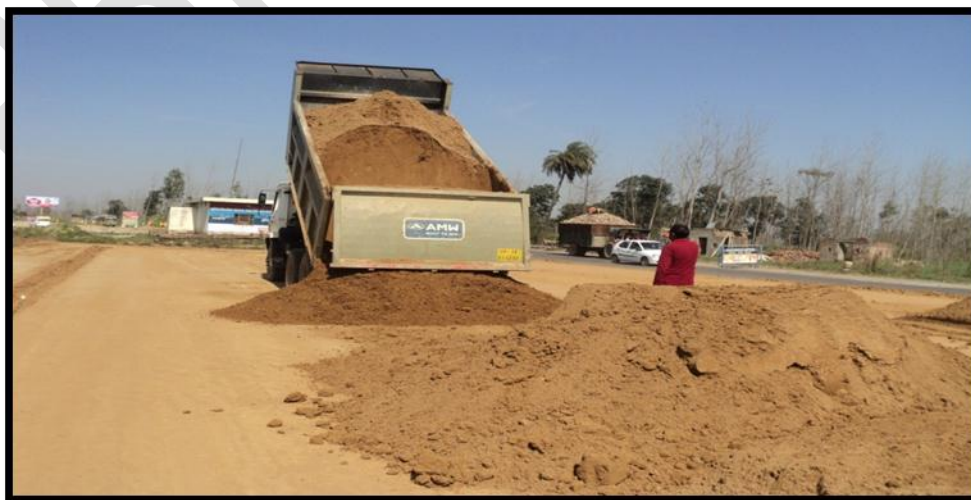
Photo 3.16: View of Dumping of Construction Material
