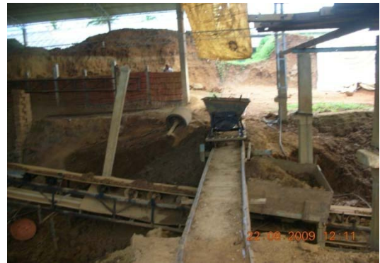
Tile manufacturing unit at Trichur, Kerala
