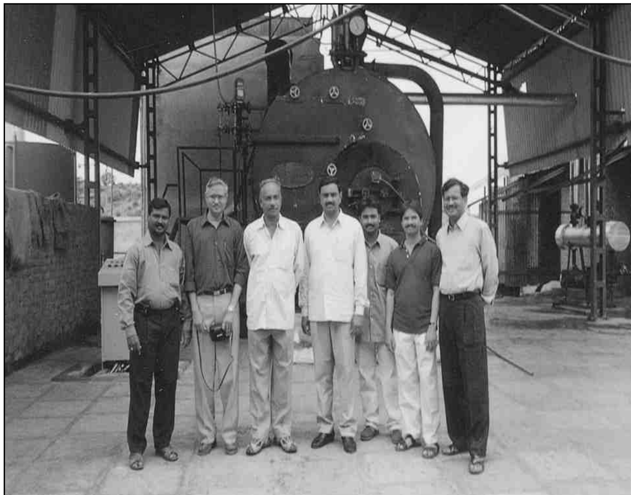
Figure 6.7 : WMC members from Raw Rice and Parboiled Rice mills at Nizamabad with WMC Facilitator Shri I.V. Ramesh Kumar having installed a new bio-mass fuelled boiler
