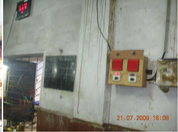
Installation of Timer (Electroplating unit, Dewas)
