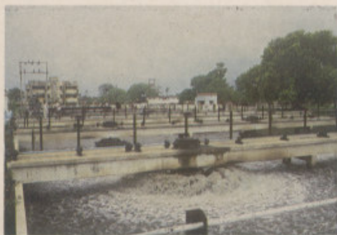
Fig 25: Aerial view of 5 MLD upflow Anaerobic Sludge Blanket (USAB) plant at Kanpur.
