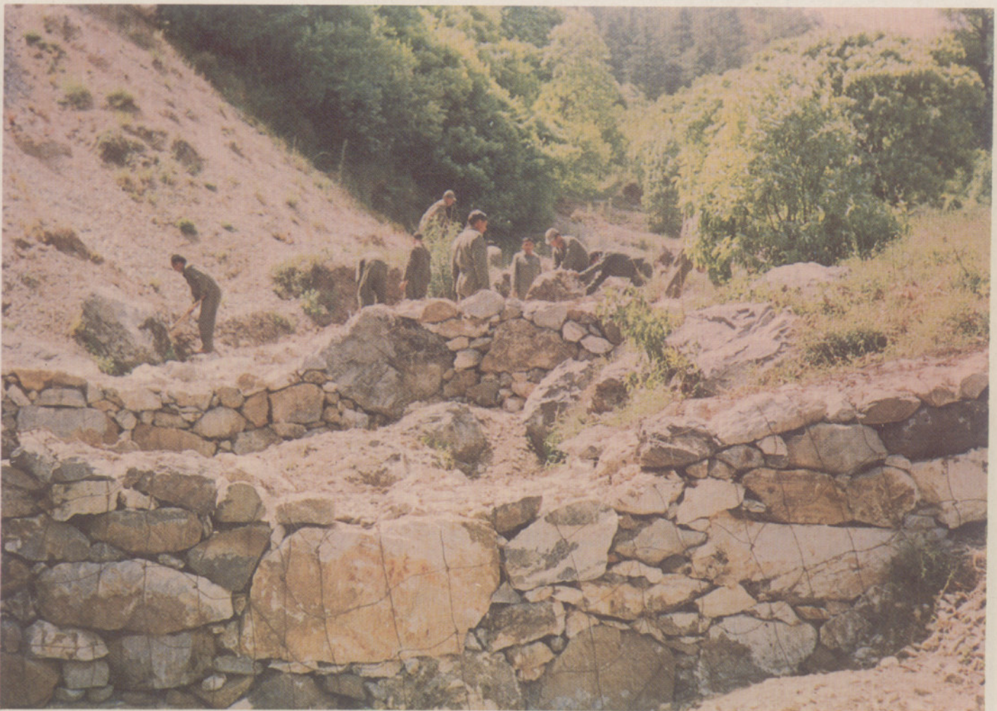
Fig. 51 Stemming Soil erosion on Mussorie Slopes by Ex-servicemen of U.P. Eco-task Force
