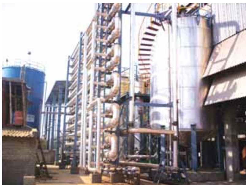
Fig-48. Lignin Precipitation System (LPS) Plant Heat Exchanger and Reactors
