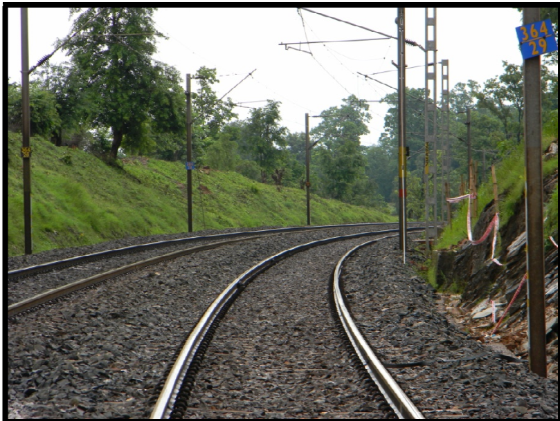
Fig. 3.8 Presence of sharp curve and embankment make the site more prone to accident (Kolhan FD)
