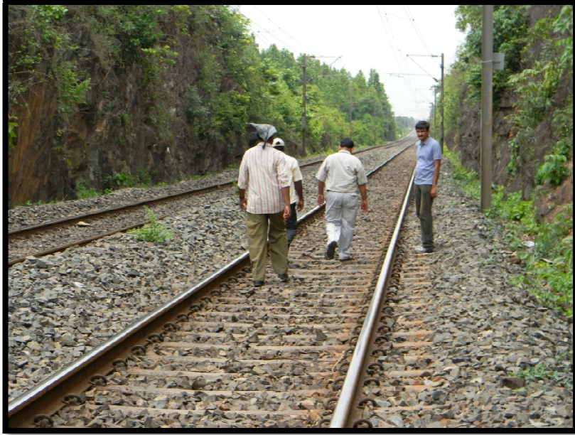
Fig. 3.7 Critical cutting at accident site in Saraikela- Kharsama FD
