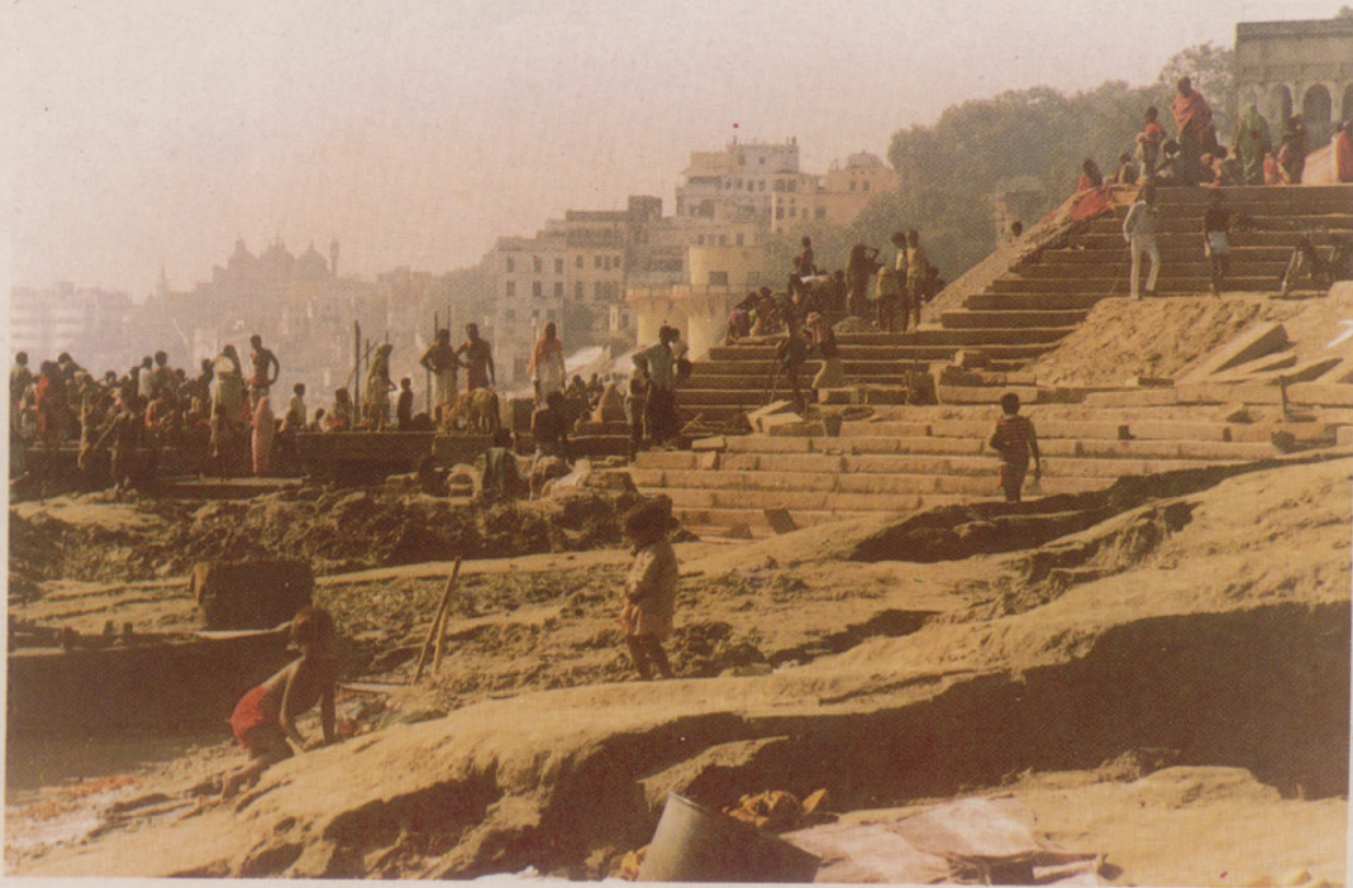
Fig. 14 Construction of steps under the integrated river front development programme in progress at Rajghat, Varanasi
