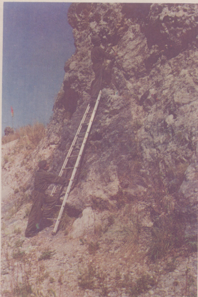
Fig. 19 Task-Force in Kiarkuli, UP, digging tube—holes on vertical mined area for planting
