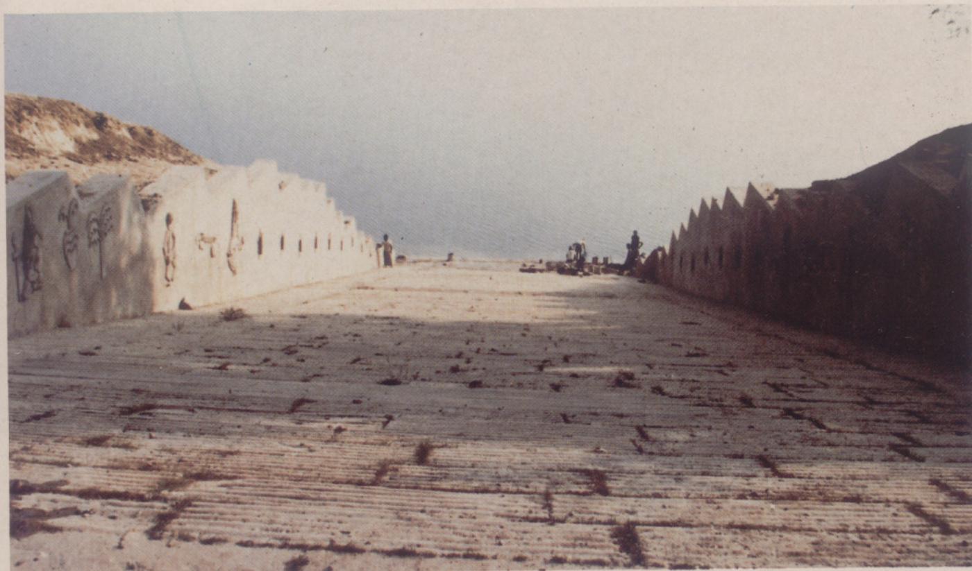
Fig 19: A view of newly constructed Saraswati Ghat, Allahabad— A River Front Development Activity under the Ganga Action Plan
