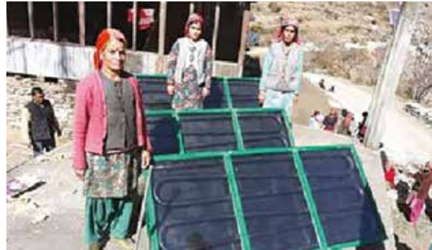
Low cost Solar Heating systems Installed at Himachal Pradesh
