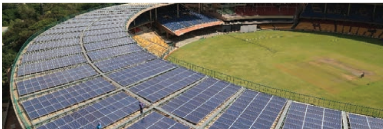
Figure 6.1: Solar rooftop at the M. Chinnaswamy Stadium, Bengaluru
