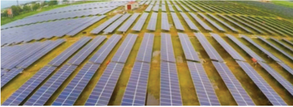
Figure 6.2: A 12 MWp solar PV power plant at Cochin International airport
