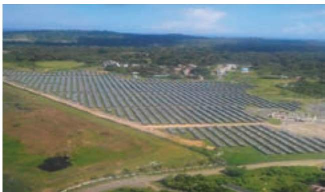
Figure 6.6: 5 MWp Solar PV Plant commissioned at Garcharma, Port Blair, Andaman & Nicobar islands
