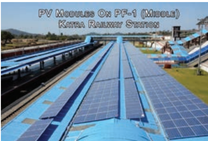
Figure 6.4: Solar rooftop power plant, Katra railway station, Jammu and Kashmir
