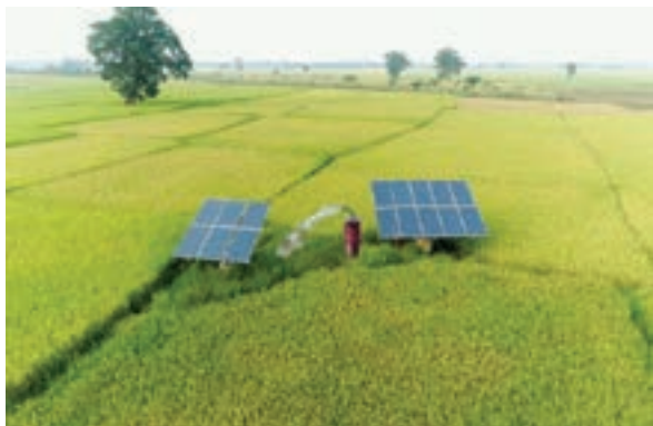
Figure 6.8: Solar Water Pumps
