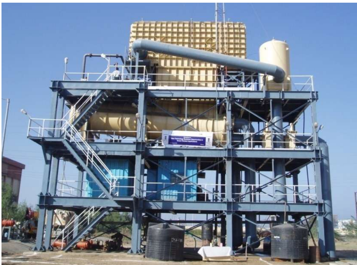
Figure 6: NCTPS desalination Plant
