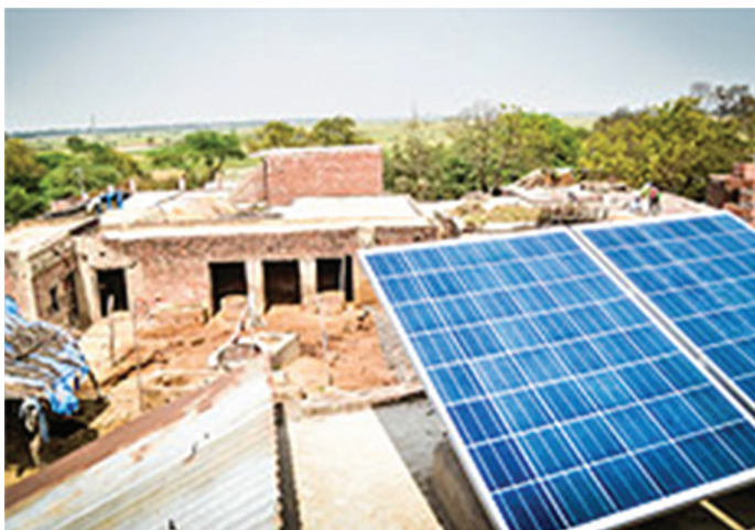
Solar Rooftop (Source: BOOND)
