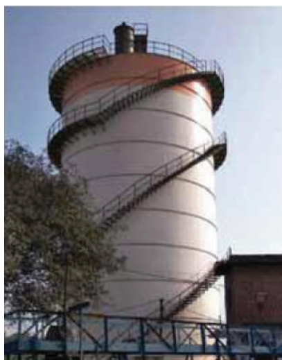
Installation of bio-digester in Paper mill as part of meeting Charter norms:
