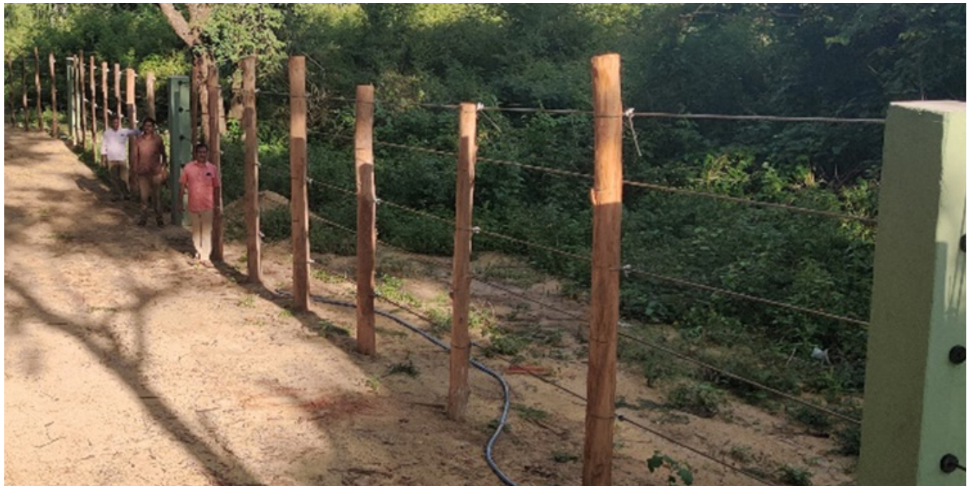
7 - Melagiri elephant fence showing precast RCC posts, steel wire rope and eucalyptus spacers
