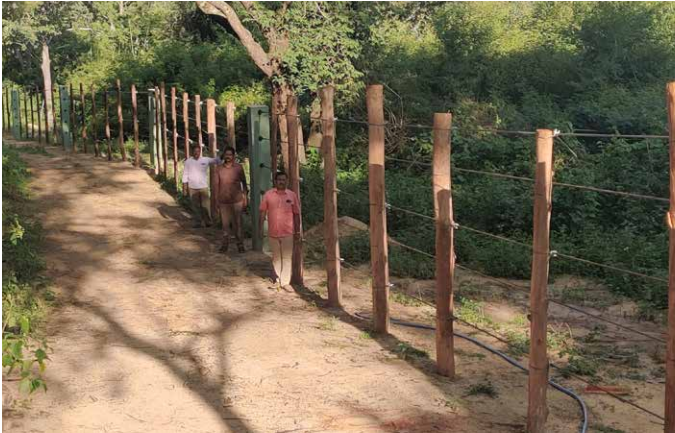
Fig 6 Melagiri elephant fence showing precast RCC, steel wire rope and eucalyptus spacers
