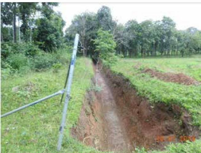
Fig 6 Trench and the solar fence in Wayanad, Kerala
