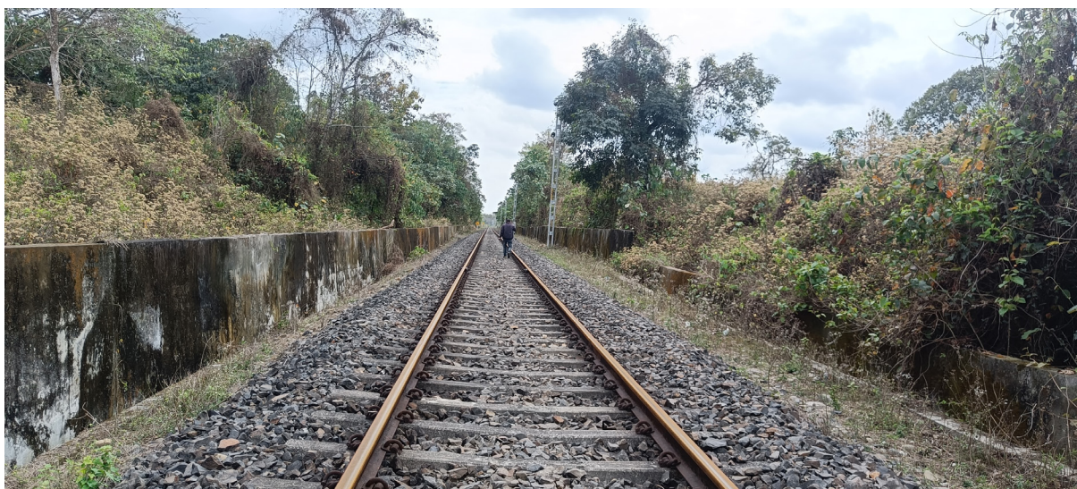
Figure 12: Concrete walls along two sections of the railway line Kalabil (Ch. 15/2 – 15/6), and that near Gamani Ban Gaon (Ch. 22/0 – 22/4) could cause elephants and other wild animals from getting stuck in the rail corridor. Multiple animal signs were found here.
