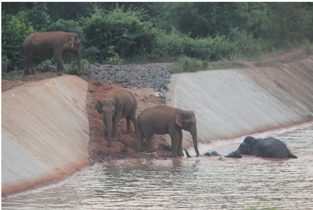
Figure 14: Ramps/exits similar to these built on canals, to facilitate escape of wild animals in the event of approaching trains in the walled sections Kalabil (Ch. 15/2 – 15/6), and that near Gamani Ban Gaon (Ch. 22/0 – 22/4) should be provided [Picture courtesy: Jagyandatt Pati]
