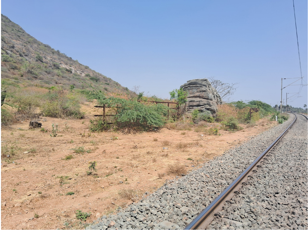
Figure 7: The old broken barriers along the Madukkarai – Ettimadai track used to stop elephants from walking on the track and crossing into the agricultural field (Chainage 498/9).
