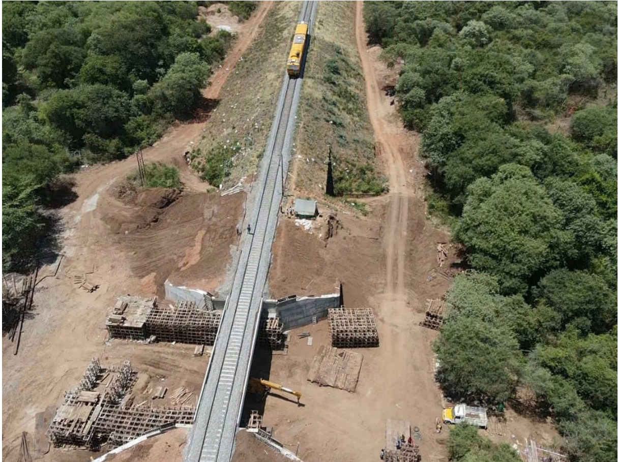
Photographs depicting the process of construction of elephant underpass on a railway line in Tamil Nadu
